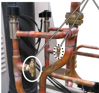
At expansion valves
